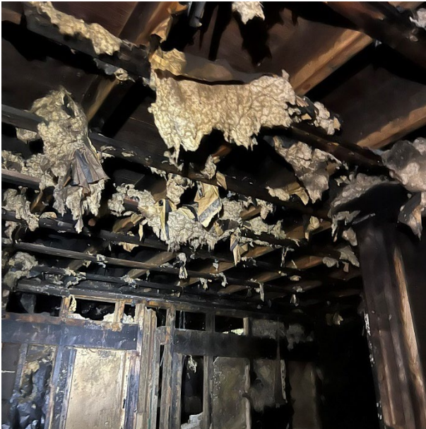
Rear Addition with Total Fire Destruction
