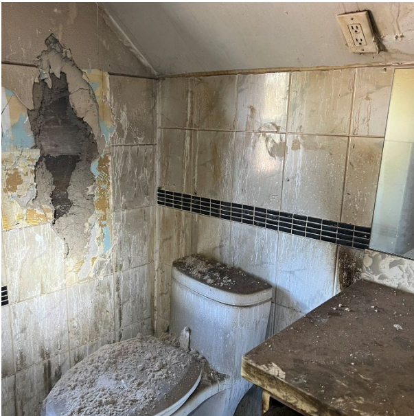
Upper-Level Bathroom with Fire / Fire Suppression Damage (Original Section)
