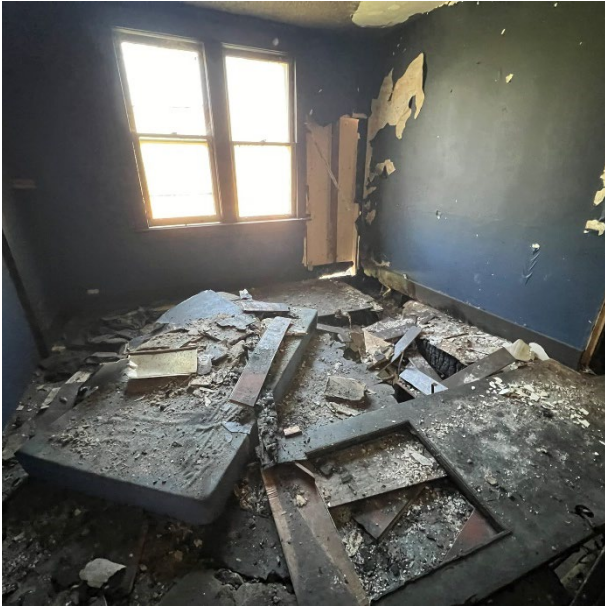
Room and Fire Damage (Original Section)
