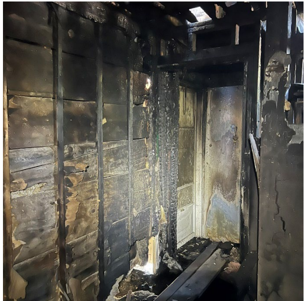
Rear Addition with Total Fire Destruction
