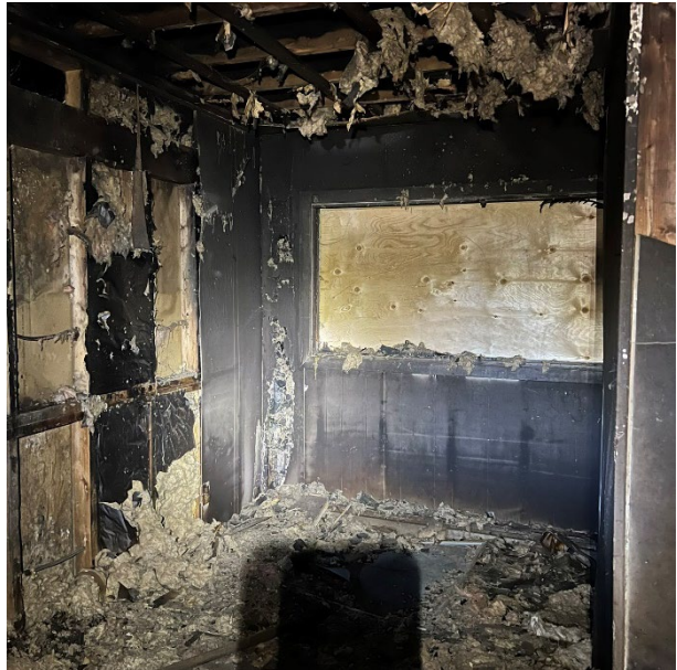
Rear Addition with Total Fire Destruction
