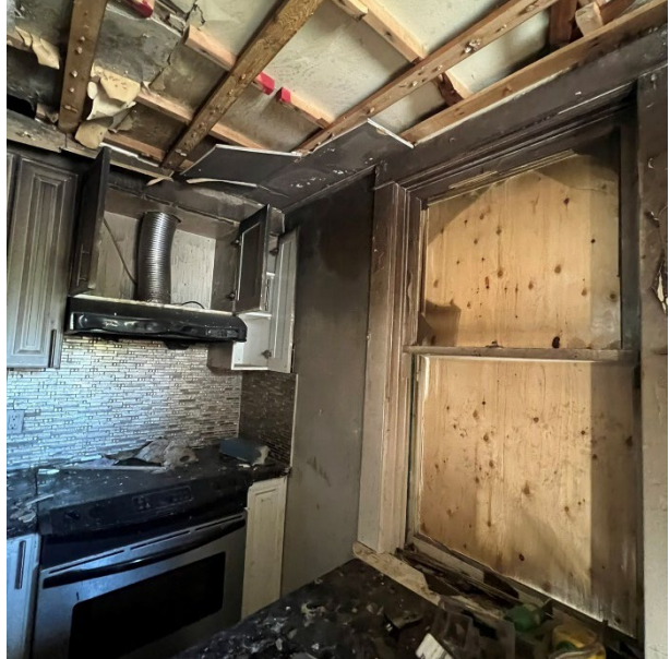
Kitchen and Fire Damage (Original Section)
