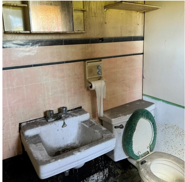
Damaged Basement Bathroom
