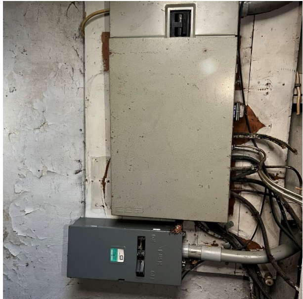
Electrical Panel (Basement)
