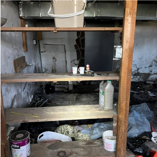
Basement with Fire / Fire Suppression Damage
