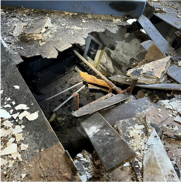
Burnt Through Floor (Basement Visible Below)
