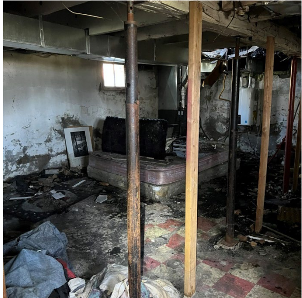
Basement with Fire / Fire Suppression Damage
