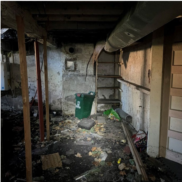
Basement with Fire / Fire Suppression Damage
