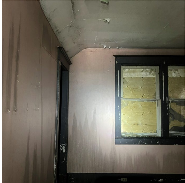
Upper-Level Room with Fire / Fire Suppression Damage (Original Section)
