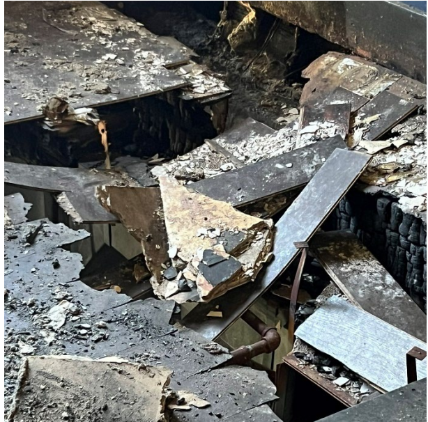
Burnt Through Floor (Original Section)
