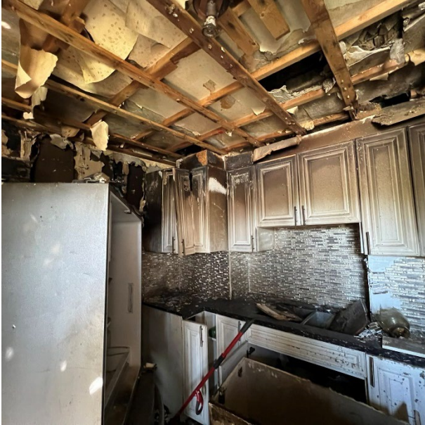
Kitchen and Fire Damage (Original Section)
