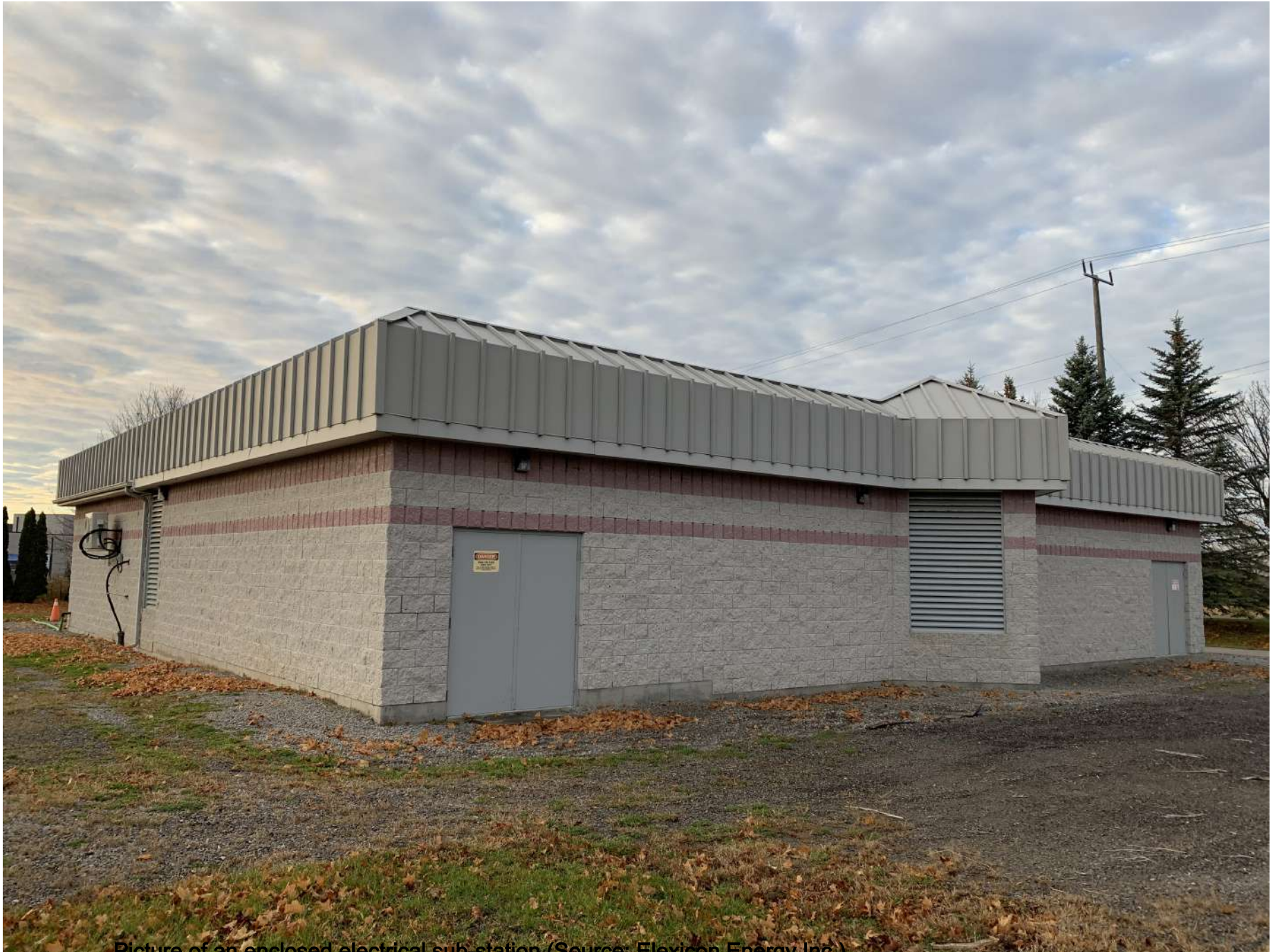
Picture of an enclosed electrical sub-station (Source: Elexicon Energy Inc.) Page 174 of 180
